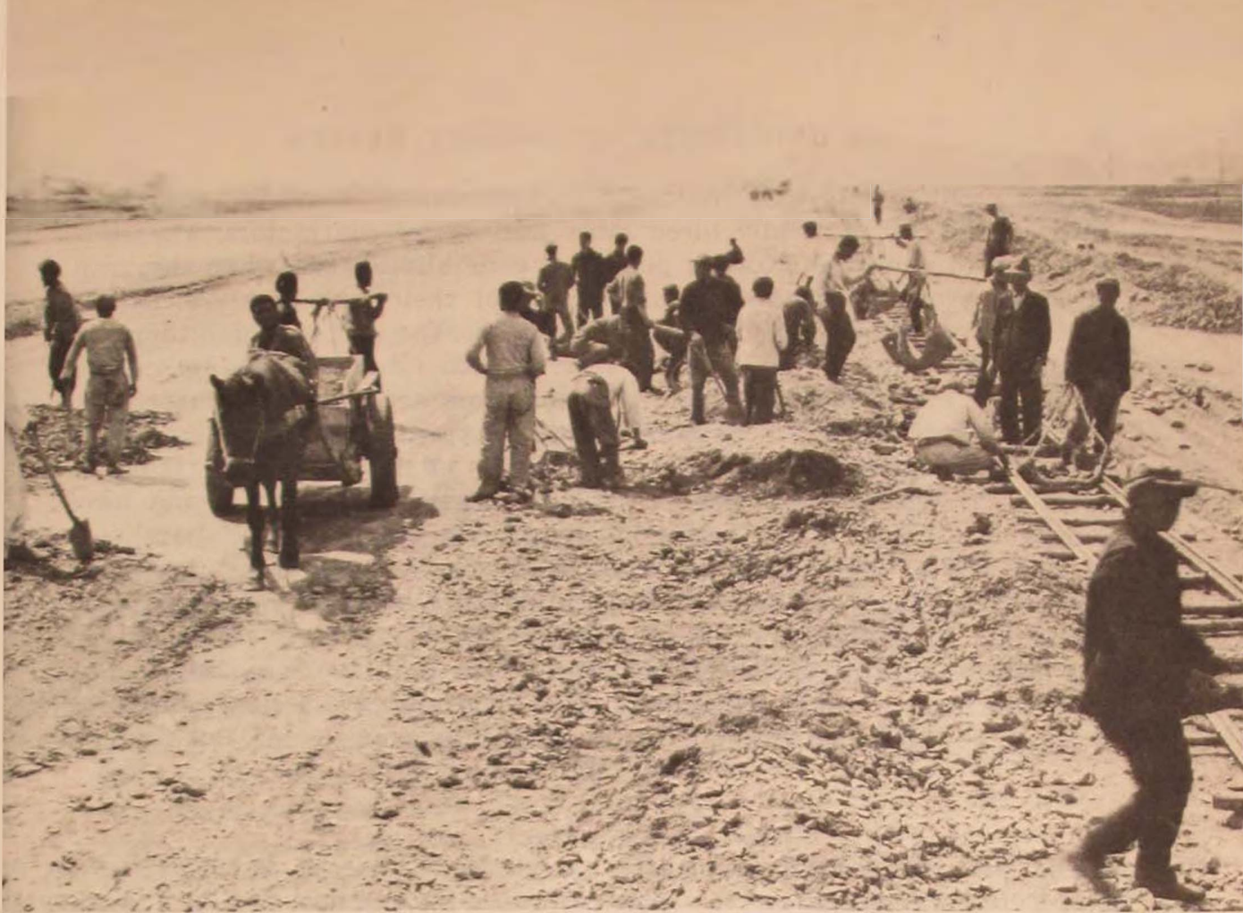
This picture of a runway construction job shows the methods used by a Korean contractor. Small rail cars bring the fill material from the quarry on narrow-gauge rail track which extends the length of the runway. Horse and ox carts, shovels, and a series of crude lift devices are used to spread the fill over the runway. The left half of the runway has been completed and is in operation while work continues on the right half.
